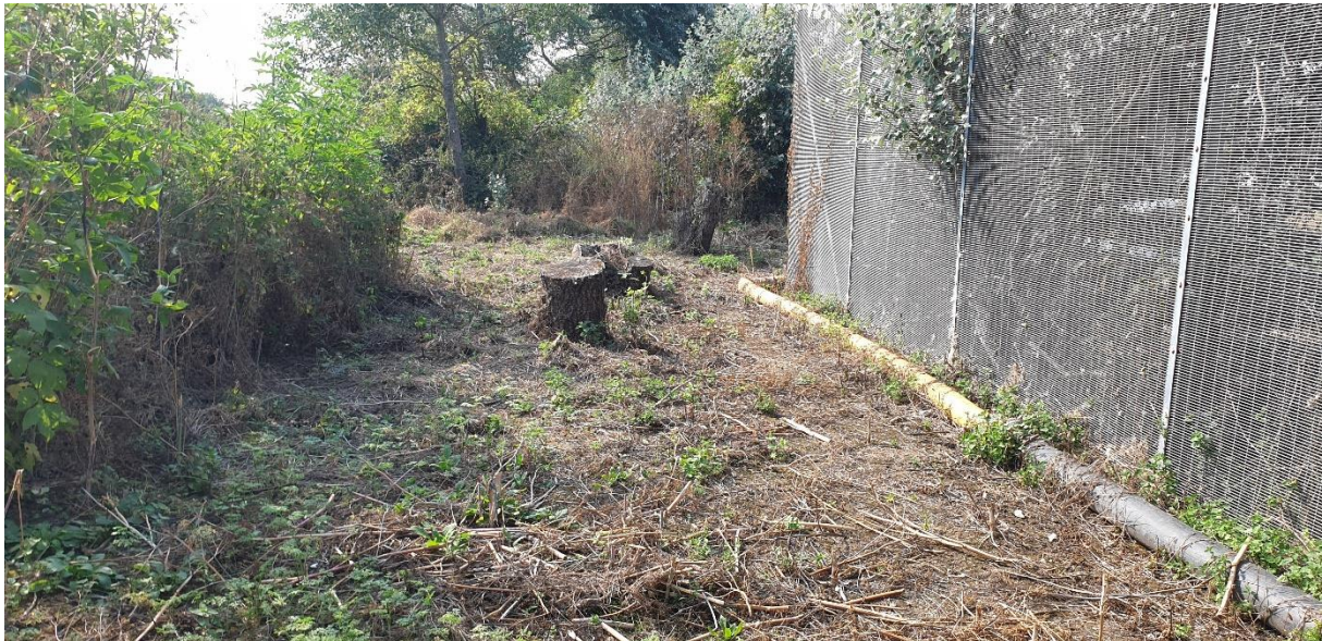
Photograph 10 – Area of woodland cleared for construction of the Keadby 2 Power Station water intake on the Stainforth and Keadby Canal
